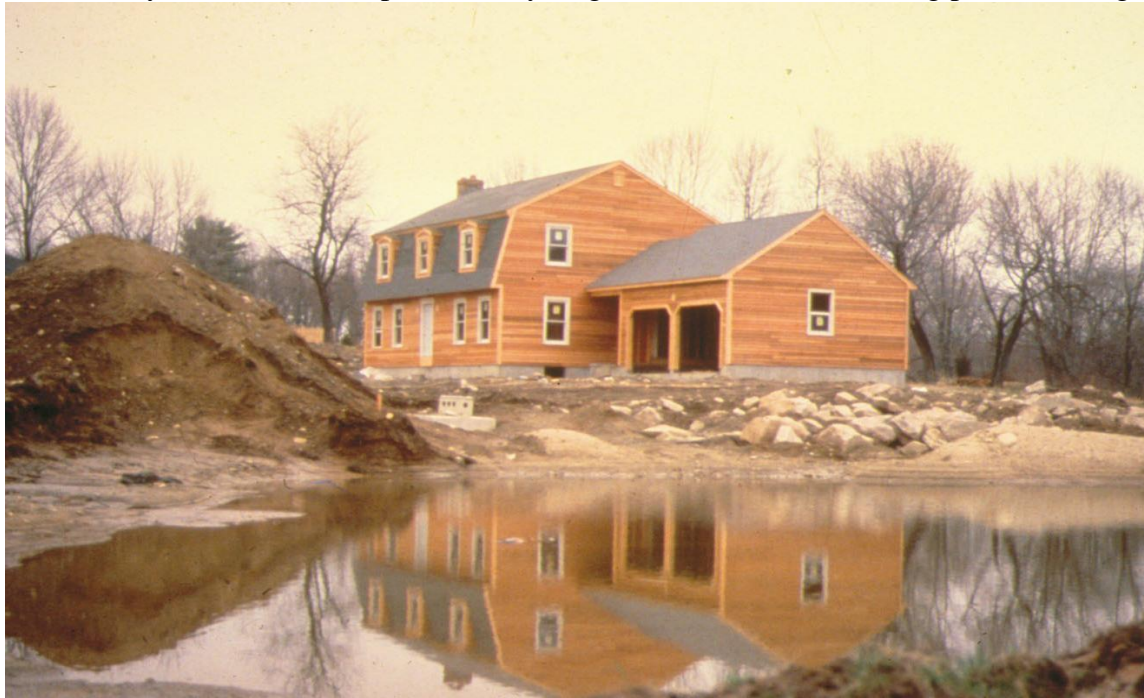
Figure 25. Septic system drainage fields will fail and basements may be wet on soils with mottled or gray subsoil and slow permeability.
