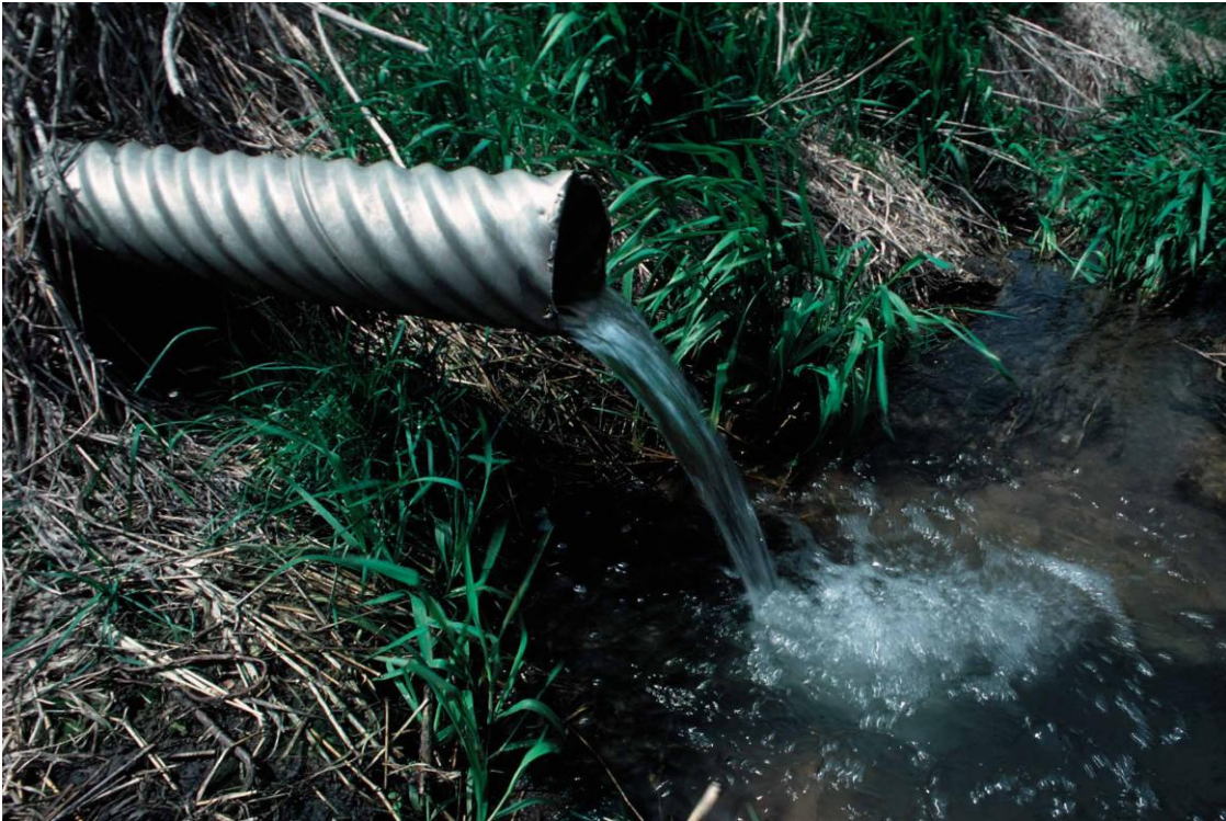
Figure 20. Outlet for subsurface drainage into an open ditch.
